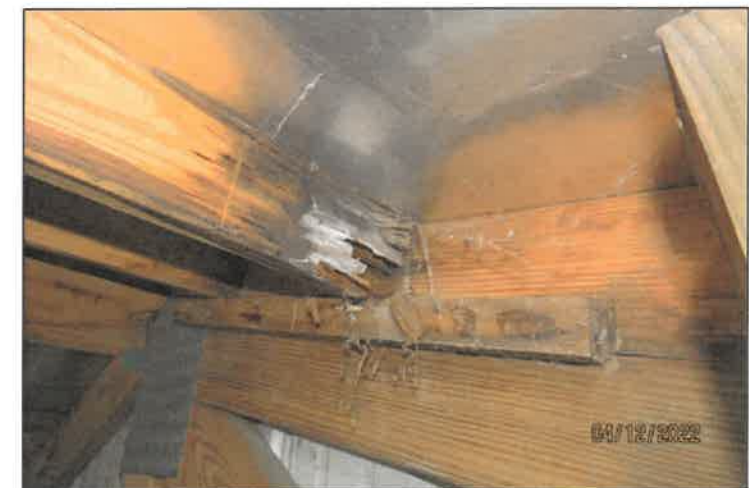
DAMAGED ROOF JOIST - STEEP SLOPE ROOF AREA
